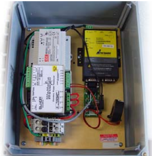
View of enclosure (without its cover) and components including communications gateway and revenue-grade meter.
